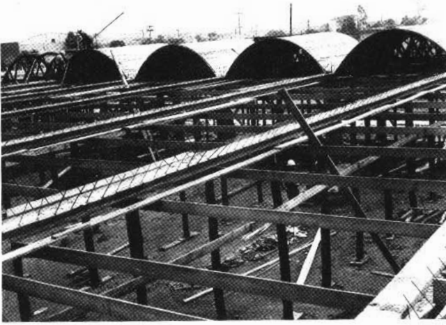
fig. 222: Small self-carrying vaults. In the foreground, the reinforced masonry "valleys" of what will be the laterally adjoining vaults can be seen; beyond, the wooden formwork for a series of barrel vaults.
