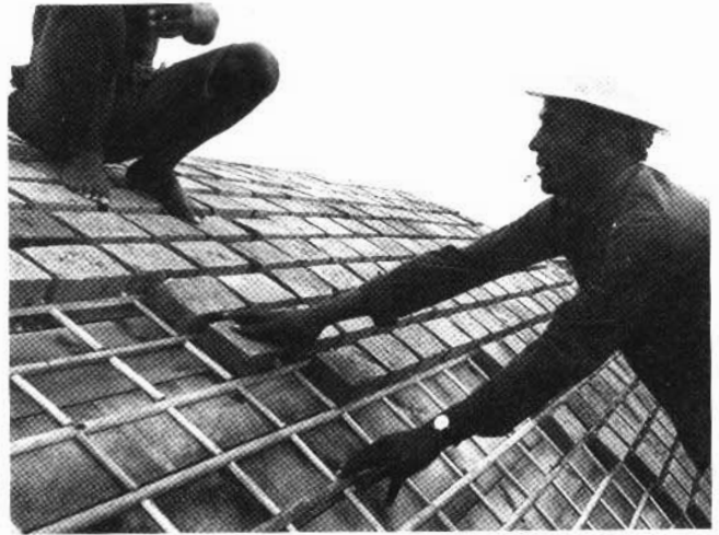
fig. 225: Small wood strips, nailed to the formwork to position the bricks. This stage is followed by the placement of reinforcing bars between the bricks and filling the joints with mortar.
