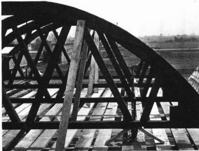
fig. 223: Timber trusses for the formwork in figure 222. The formwork moves on rails set on the timber platform.
